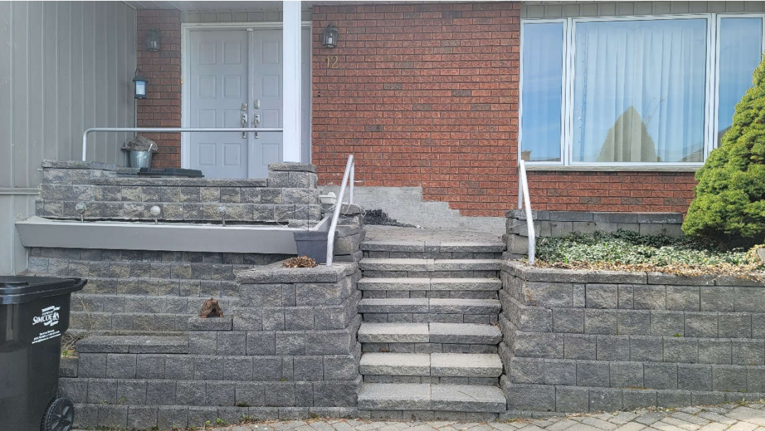
Existing use in Need of repair / Note damage/ sinking due to underground water
