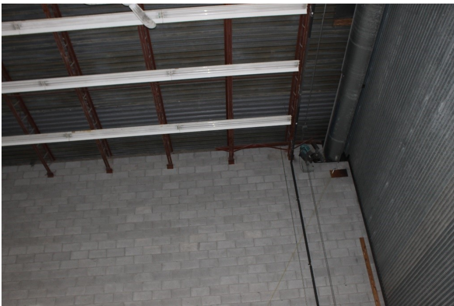
Photograph 2. Interior of large boat workshop at the north end of property. (September 25, 2018)
