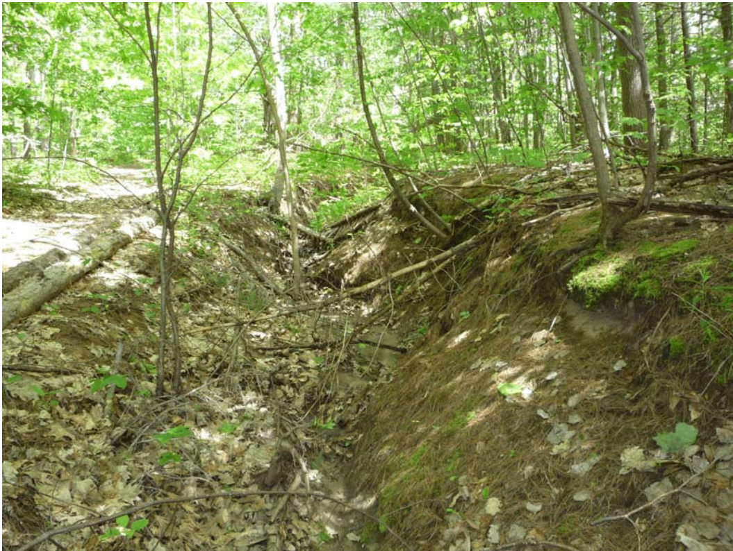
Photograph 8. Erosional gully, from uncontrolled stormwater from east (August 9, 2010).
